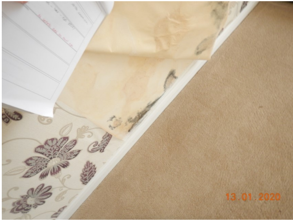
Damp to most walls
