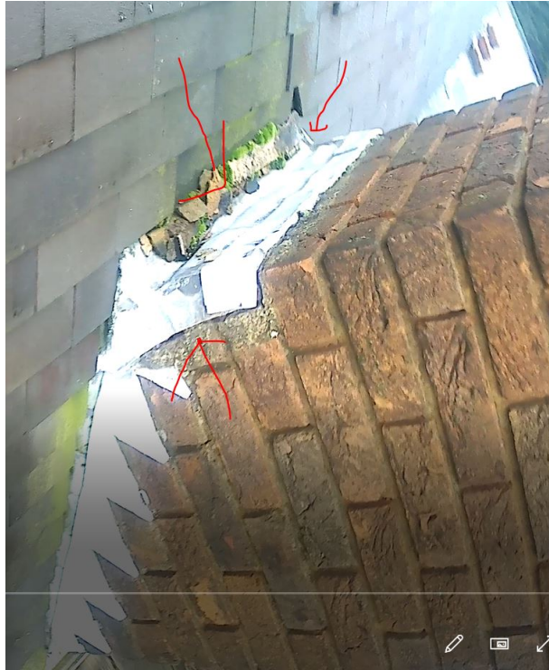
chimney flashings need attention
