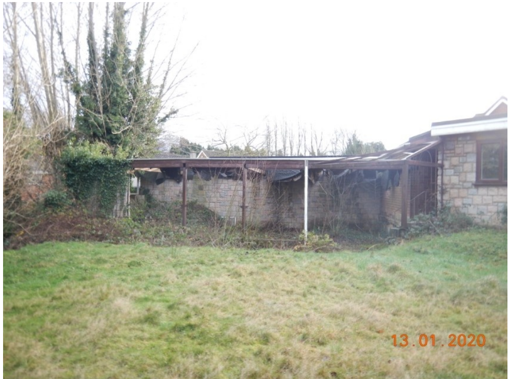
derelict metal frame structure
