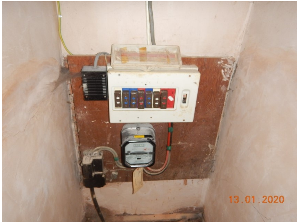
old fuse board
