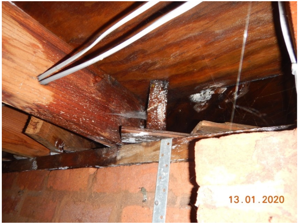
rot caused by leaking flat roof
