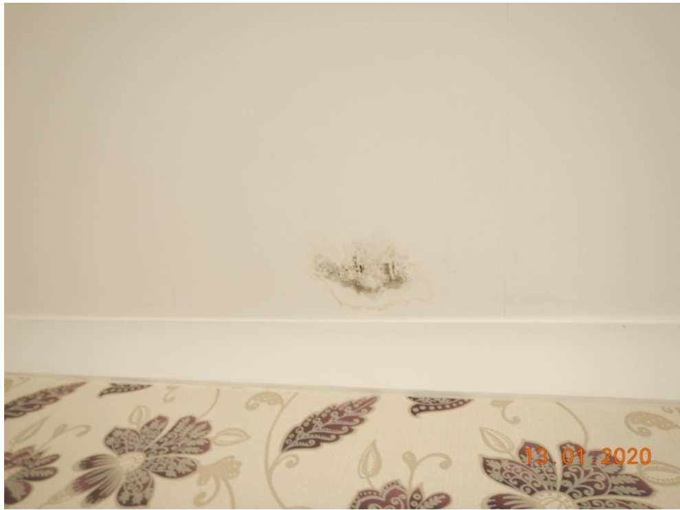
mould due to rain ingress from right hand chimney
