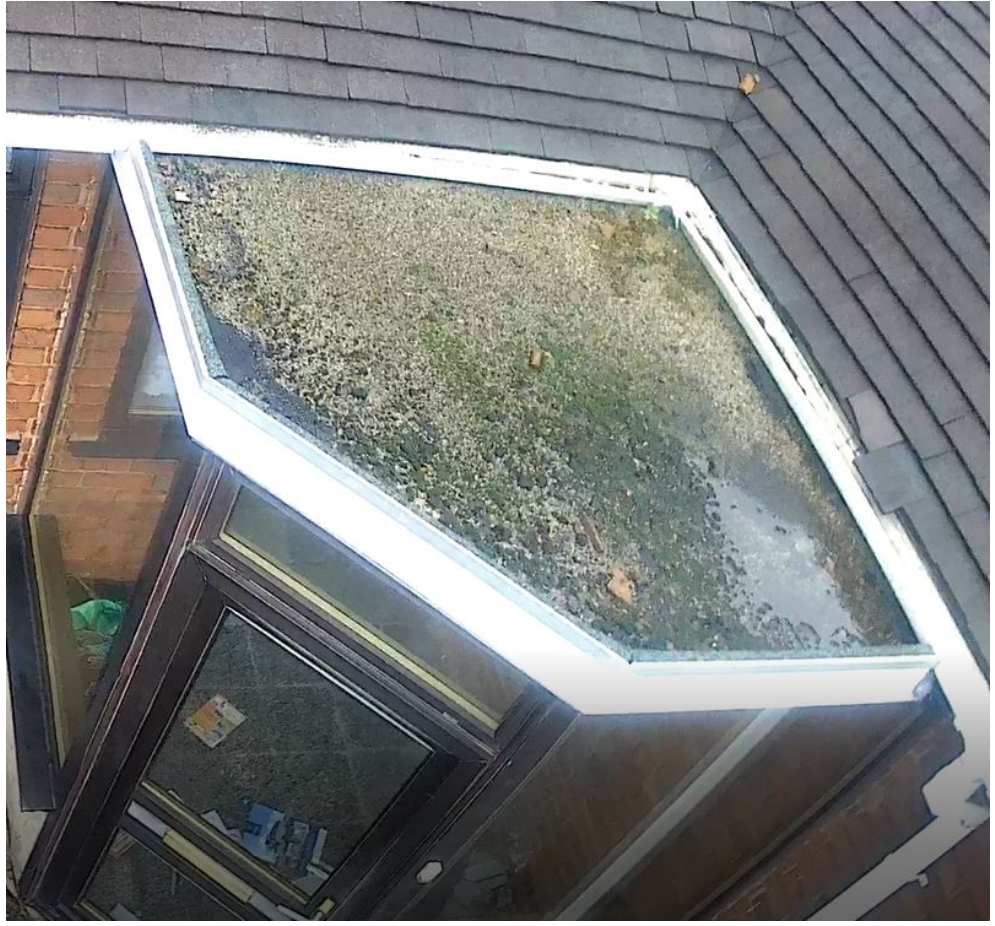
porch roof needs renewal
