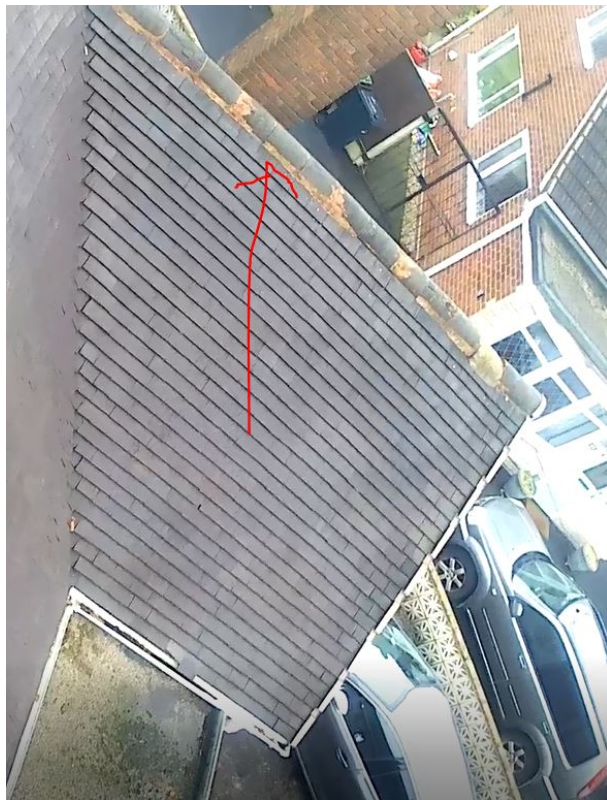
ridge tiles need renewal
