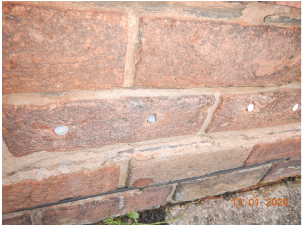
conventional DPM and retro chemical injection
