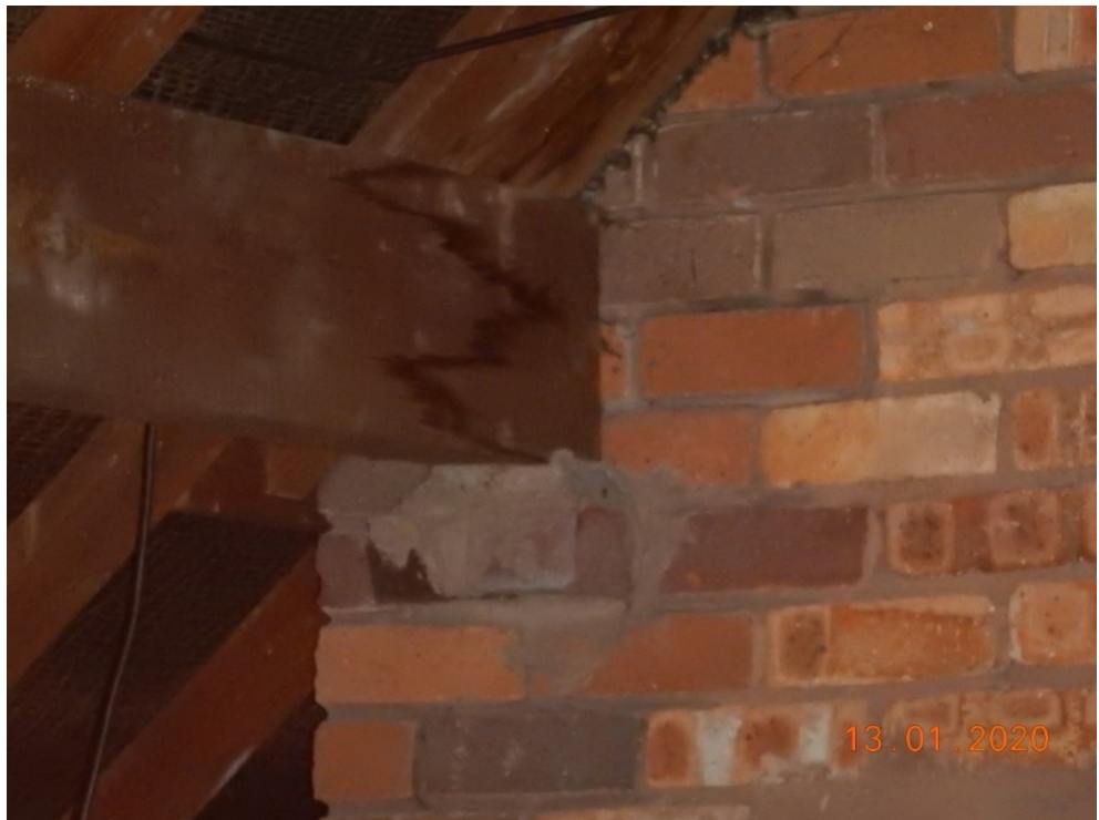
Staining to timber around chimney
