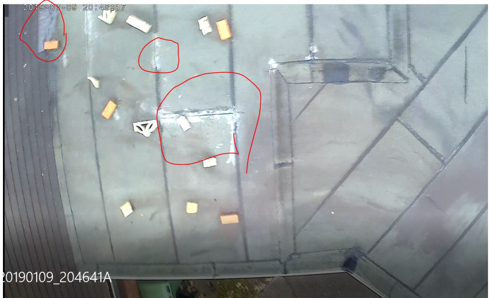
flat roof poor repairs
