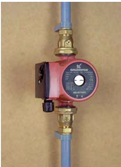
Connection to pump
