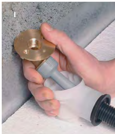
Conduit Terminal body fixed to floor. Pipe within conduit then push-fitted into retaining cap of brass connecting plate.
