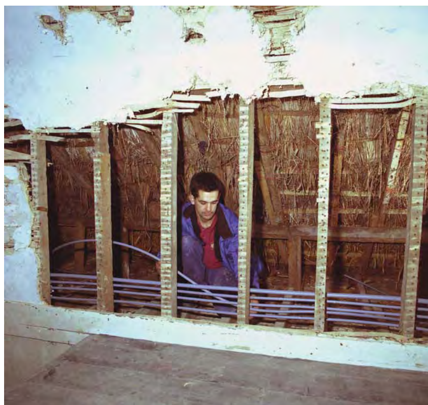
Flexibility and push-fit joints ease installation and ensure safety in the restricted space under the eaves of the thatched roof
